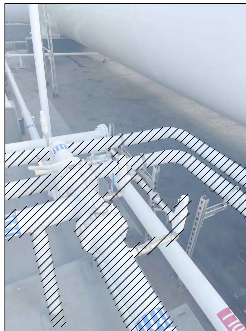
H TANKS #6 & #7 MANIFOLD - LOOKING NORTHEAST SCALE: N/A
