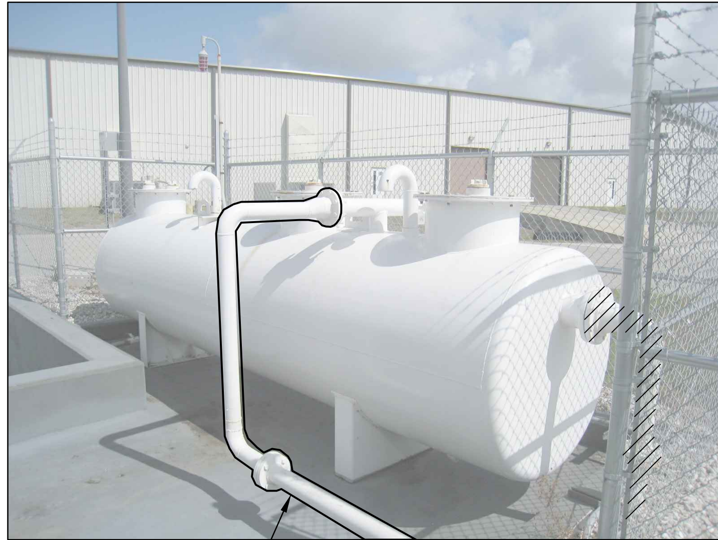
(E) PIPE AND SUPPORTS TO BE TEMPORARILY RELOCATED TO SUIT RELOCATED OWS, SEE FM1.05A, FM1.05B & FM2.10
