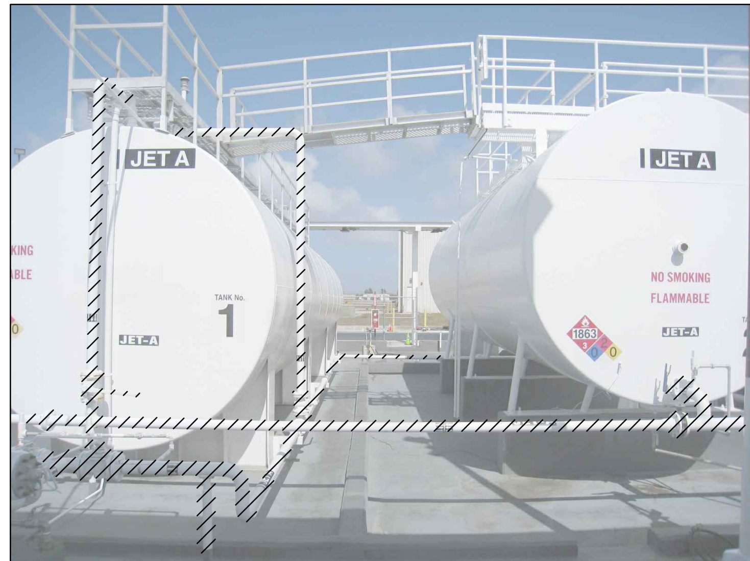
D TANKS #1 & #2 - LOOKING NORTH SCALE: N/A
