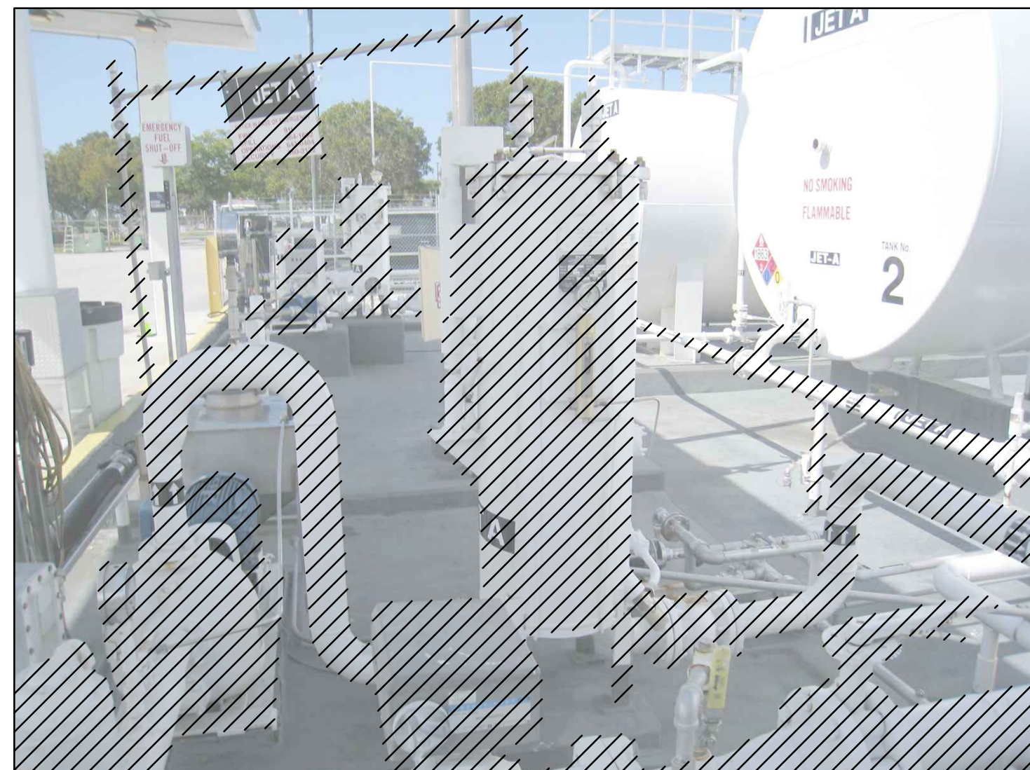
G FILTER SEPARATOR #2 - LOOKING WEST SCALE: N/A
