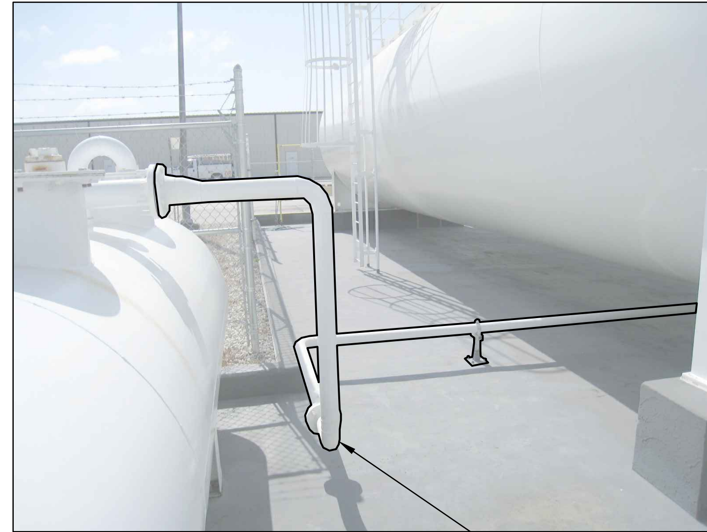
(E) PIPE AND SUPPORTS TO BE TEMPORARILY RELOCATED TO SUIT RELOCATED OWS, SEE FM1.05A, FM1.05B & FM2.10
